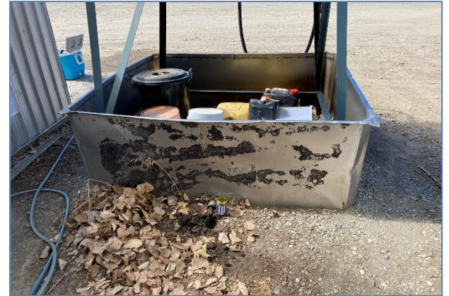
Photo 9: Outlet of the bunded area beneath an above ground fuel storage tank.
