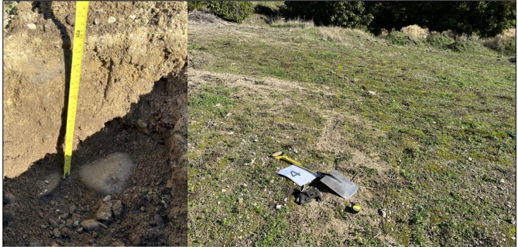
4. Fill with no topsoil present over stones and gravel.
