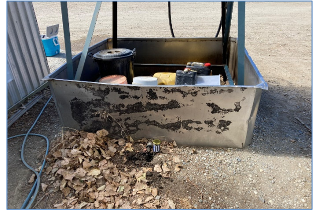
Photo 9: Outlet of the bunded area beneath an above ground fuel storage tank.
