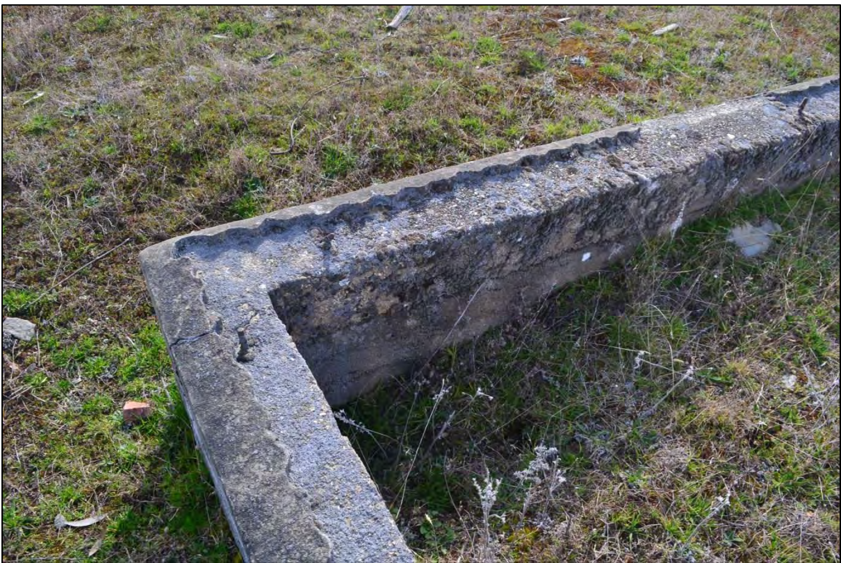
Figure 8. Detailing of concrete house foundation showing steel bolts and remains of cast plaster on exterior edge, indications the original cladding was corrugate iron.
