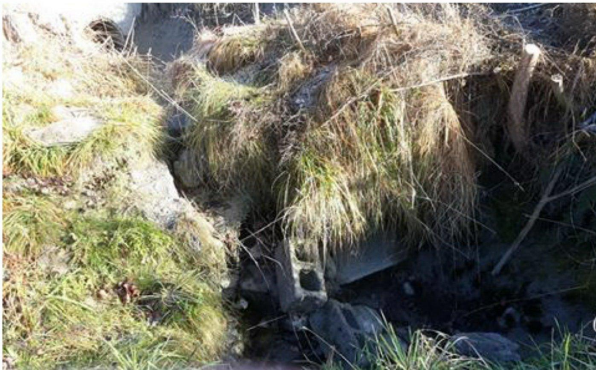
Damage to the main A and B race junction
