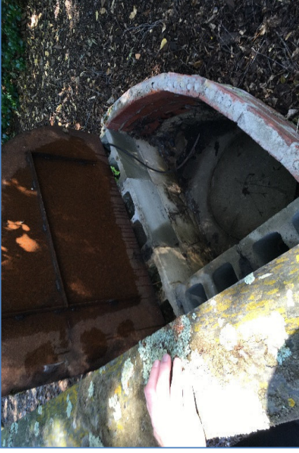
Photo 21: Underground water storage tank, south of the dwelling on the southern property.
