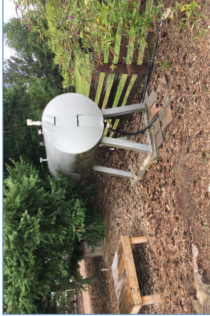
Photo 16: Above-ground fuel storage tank on the southern central property.
