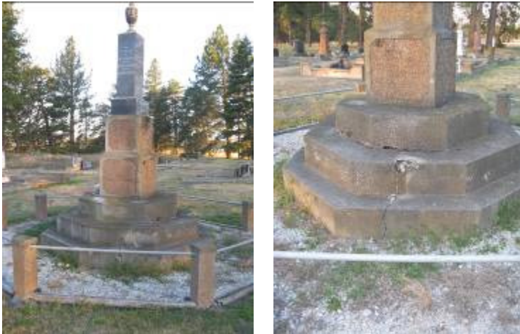
Photos M 3 & M4 – War memorial on lean and concrete base damage
