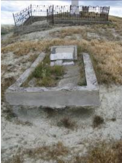
Photo V8 - Showing undermining of graves
