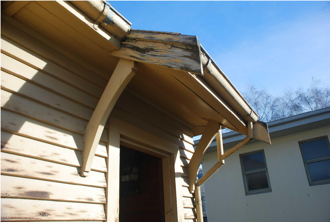
Figure 27 The canopy roof over the entrance door supported on painted timber brackets.
