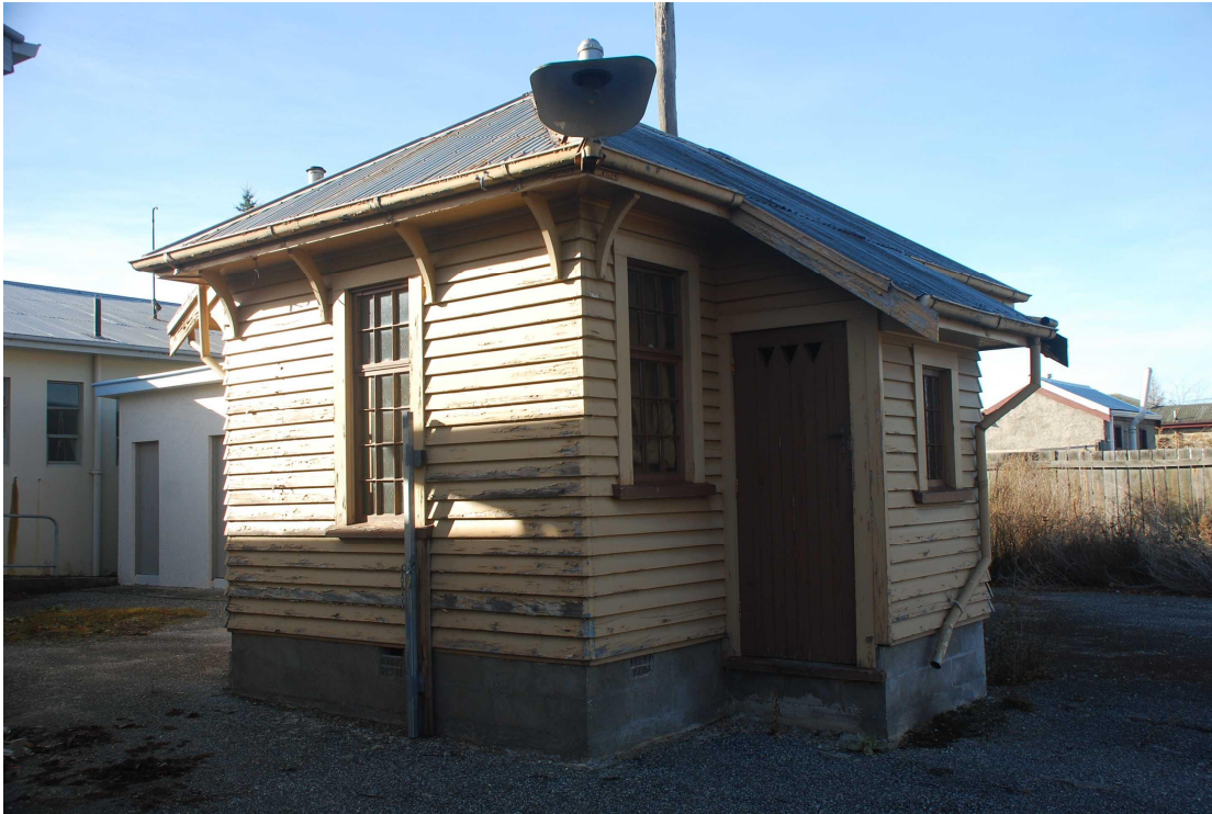
Figure 17 The side and part rear elevation. The left and centre windows light the lobby and the lean-to projection has a small rear window and vented timber door. The lean-to which provided a WC is only accessible from the exterior of the building.
