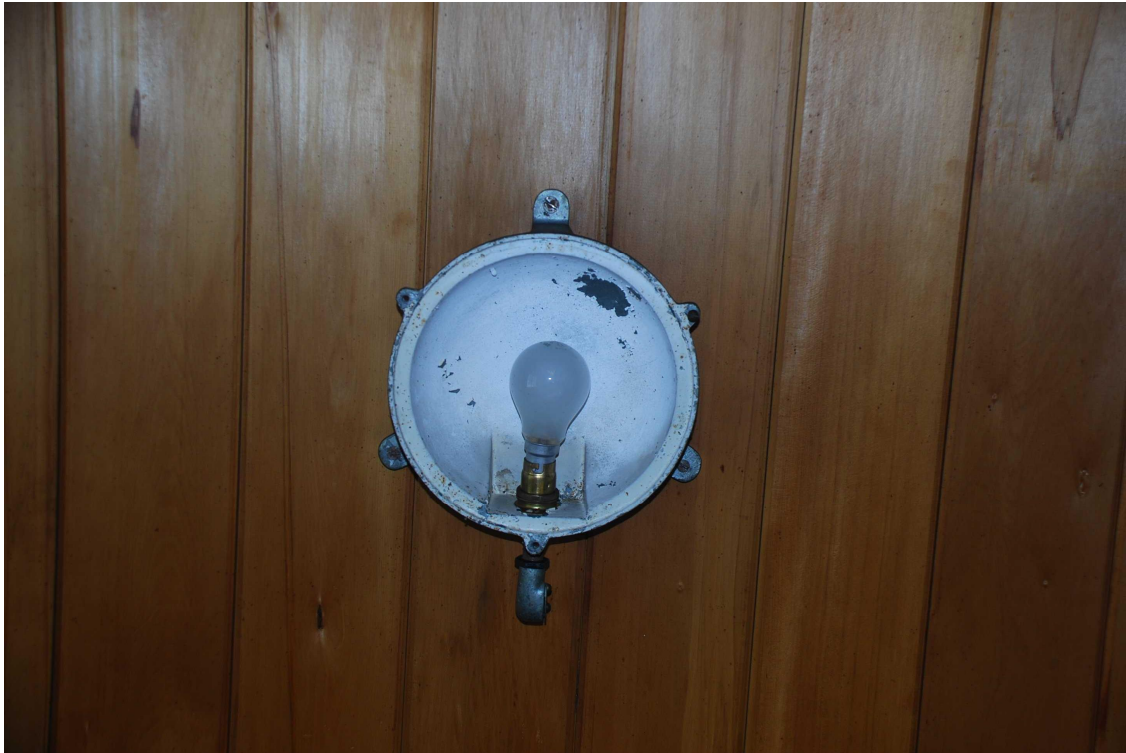
Figure 37 Steel bulkhead light fitting.
