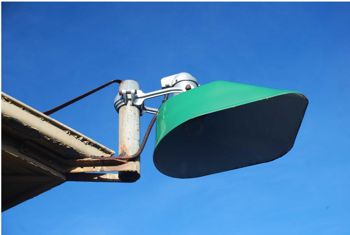
Figure 38 External floodlight at roof level to the rear external corner of the lobby.
