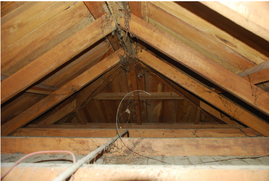
Figure 20 The roof void above the cell (a small ceiling hatch is provided in the lobby).
