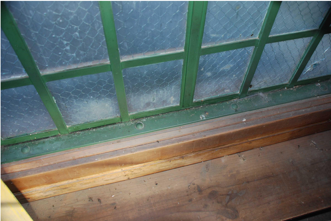
Figure 24 The interior of one of the two cell windows showing how the window is bolted into the framing.
