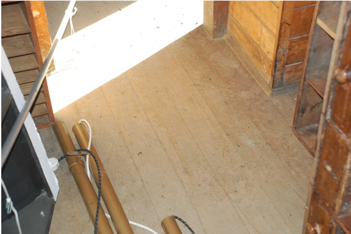
Figure 35 Tongue & groove flooring in the doorway of the cell (looking into the lobby).
