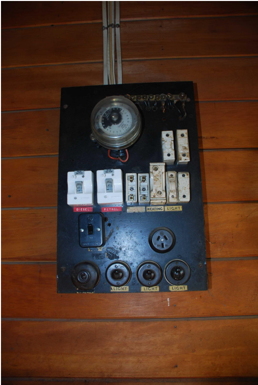
Figure 33 The fuse board with old light switches and more modern fuses.
