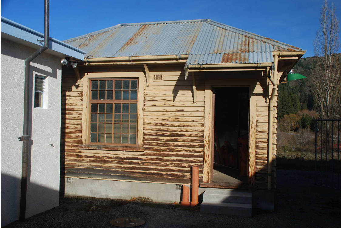
Figure 16 The front elevation with galvanised steel clad hipped roof and projecting canopy over the entrance door; painted, timber shiplap weatherboards; galvanised steel rainwater fittings; eaves brackets; and large, rectangular cell window of galvanised steel with fluted and wired glass. The entrance door leads to a lobby running the depth of the main building.
