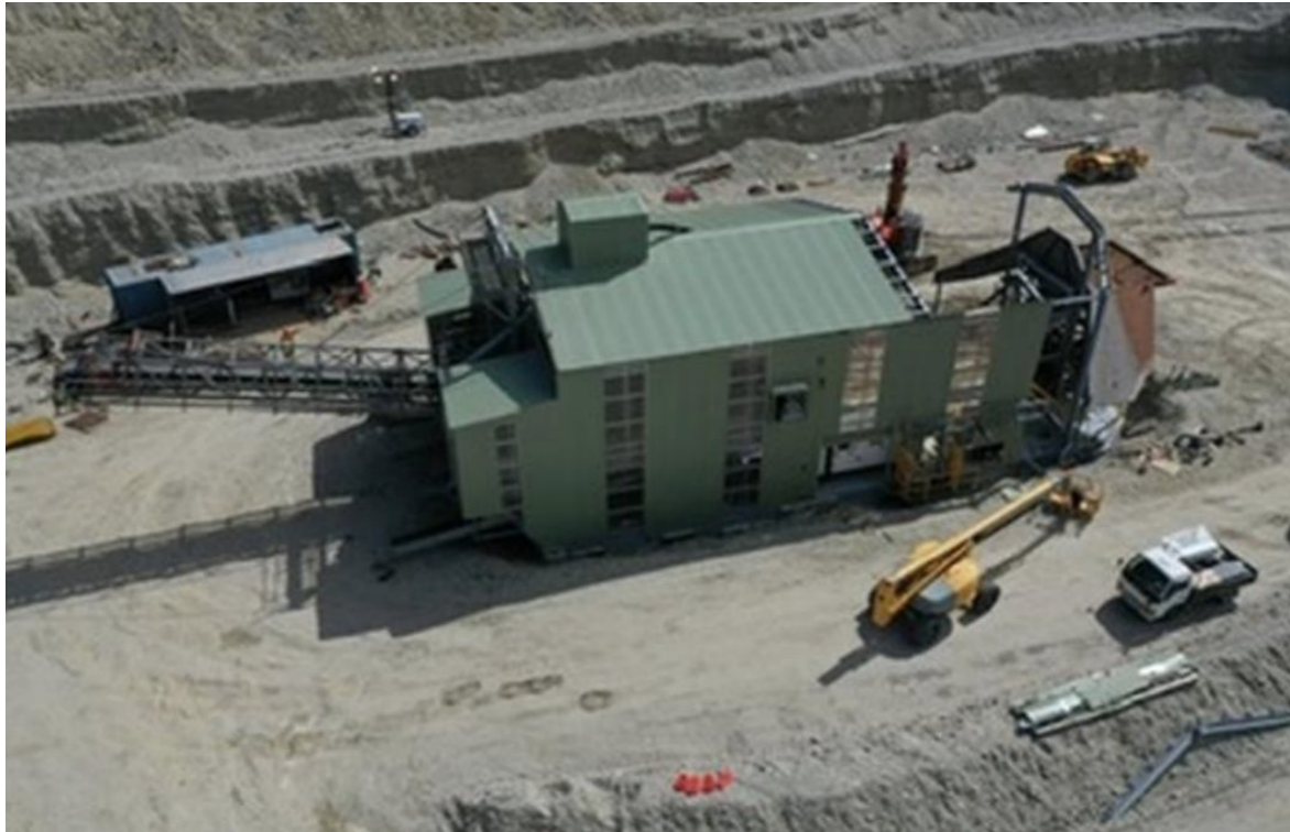
Figure 3: The Gold Recovery Plant. Source: Further Information Response
