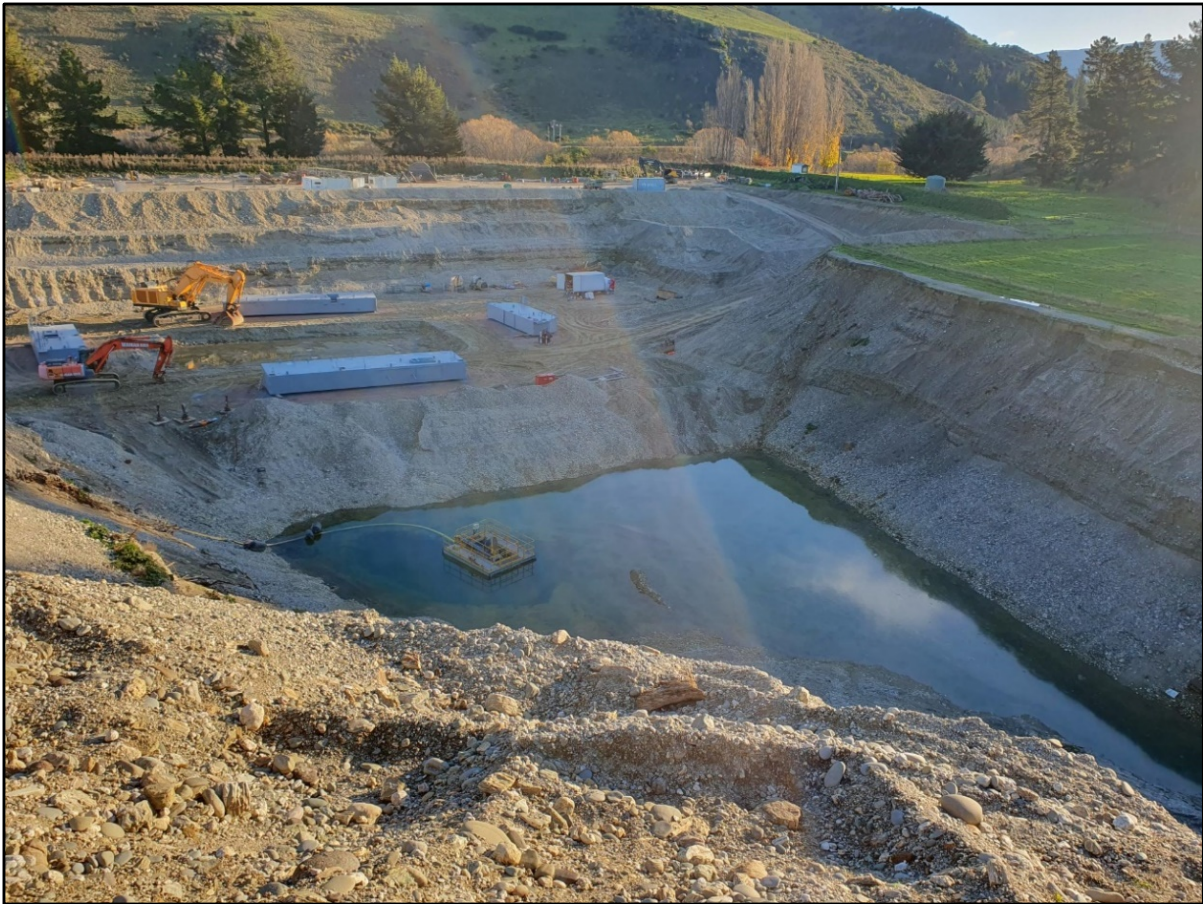
Figure 5: Works already undertaken on the site. Source: Council compliance site visit photos taken on 15 May 2023.
