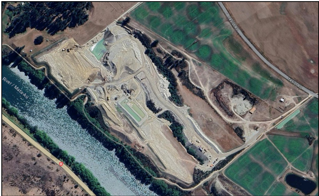
Figure 6: Aerial photo of the works undertaken on the site. Source: Google Maps, Screenshot taken 11 March 2024.
