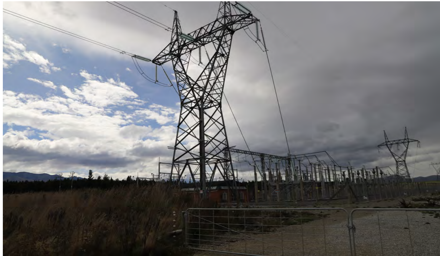
Site Context Photograph 11: View from Fennessy Road to the existing substation, approximately 1.8 kilometres northwest of the Site.
