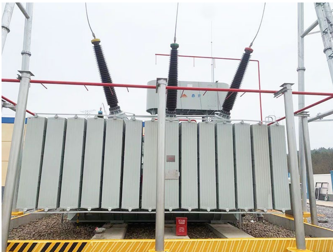
Image 3: 150MVA 33/220KV transformer
