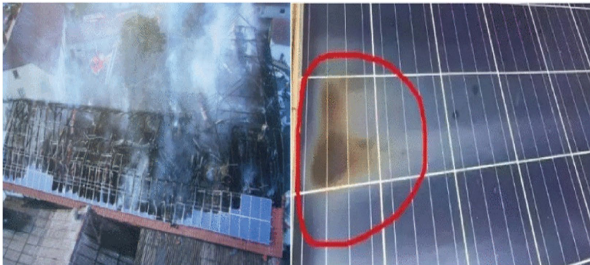
Image 1 Fire initiated by a hotspot in a PV panel
