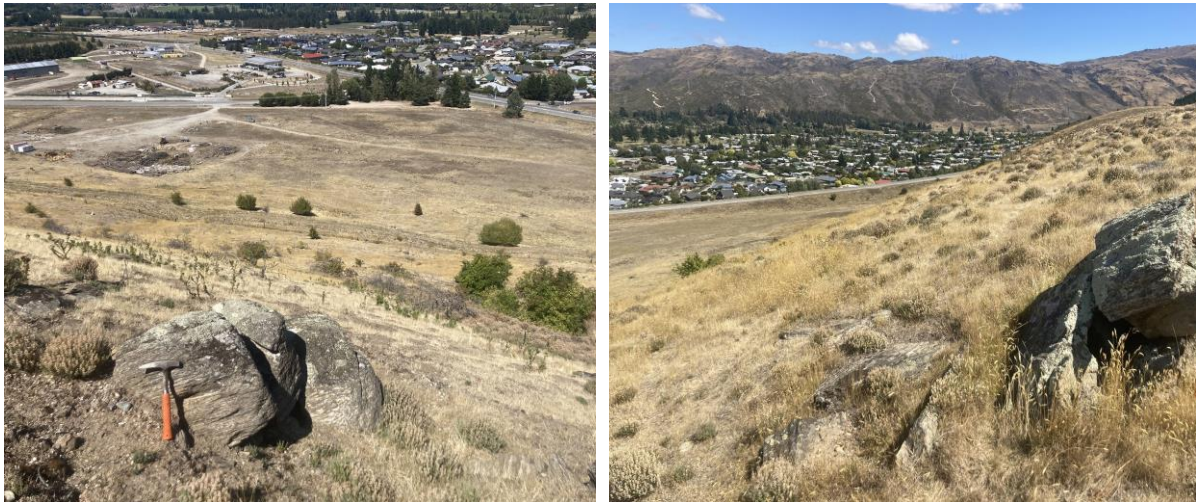
Photos 3 & 4. Example boulders with the most potential to become dislodged from the terrace slope. Geological hammer for scale.
